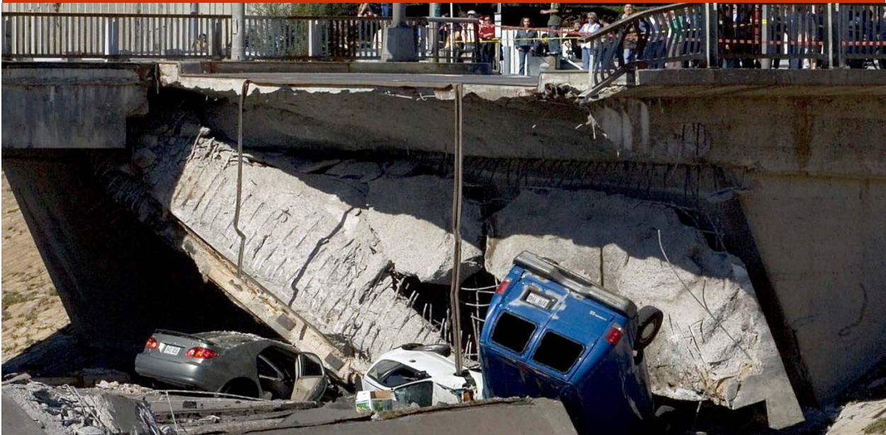
Figure 6: 2006 Quebec De la Concorde Overpass collapse resulted in 5 deaths, 6 injuries
