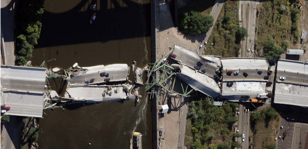
Figure 5: 2007 Minneapolis I-35 Bridge collapse resulted in 13 deaths, 145 injuries
