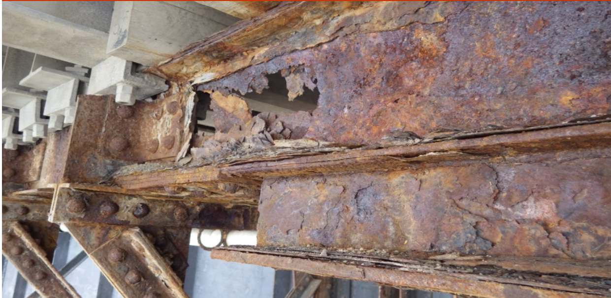
Figure 8: Inspection photo of a bridge girder given a “poor” condition rating
