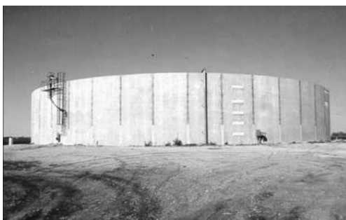
Above-ground concrete manure storage facility
